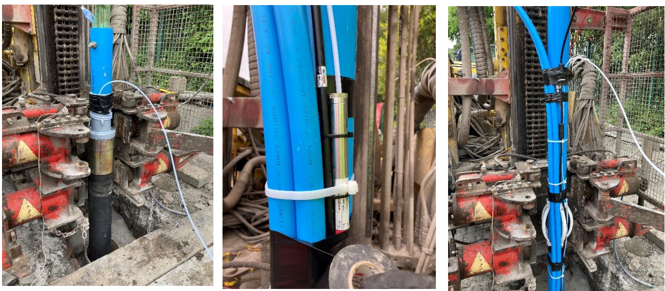
Fig. 10: Image acquired during the installation of the 4" casing and adjoining cables completed in June-2023
